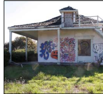
February 2012 - Moraga Adobe with lots of graffiti. Photos by Kent Long
